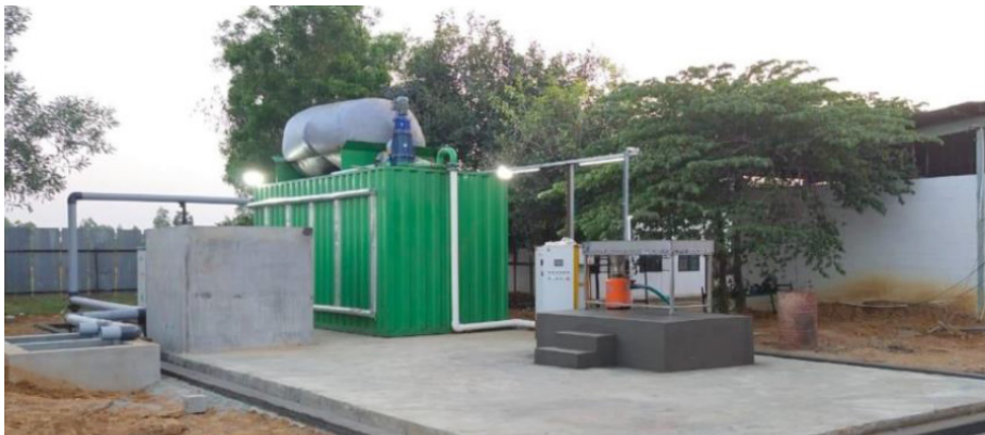
Figure 12: Container AD solution “Bert Mobil AD”. [8]
